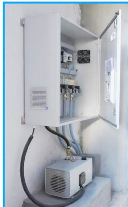
ALL ELECTRICAL PARTS KEPT OUTSIDE
