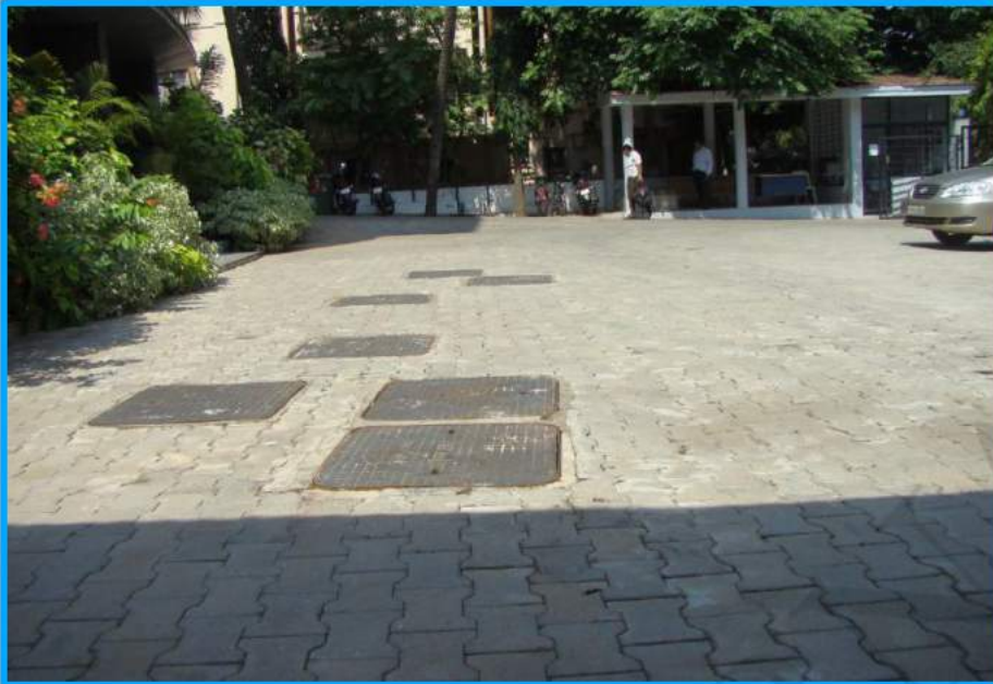
STP TANK PLACED UNDER THE WALK WAY IN D&B OFFICE CHENNAI
