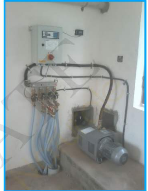
THE CONTROL ROOM OUTSIDE
